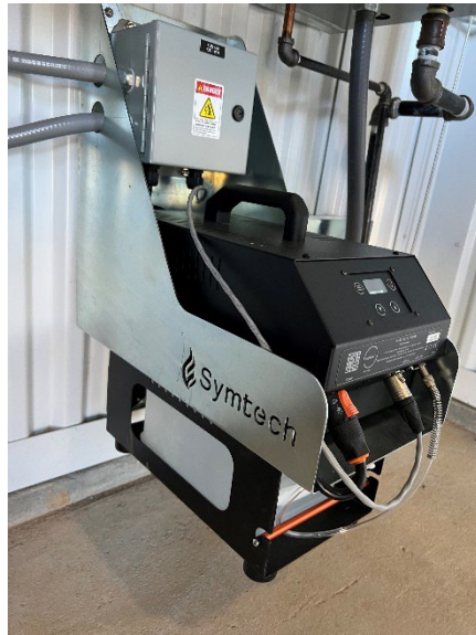
Dedicated 70,000 cfm Burn Room Smoke Machine (1 Per Burn Room)
